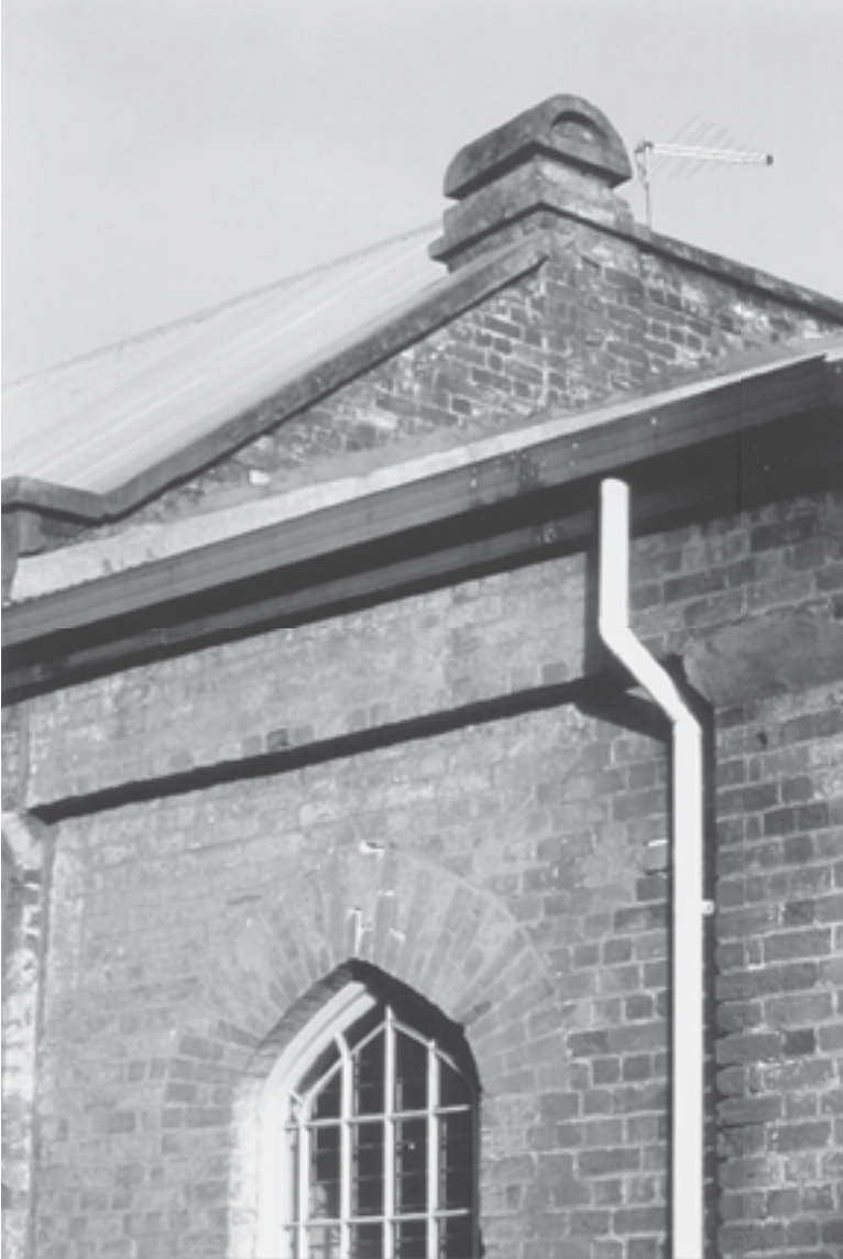
Figure 4. A 'Soane's knob' finial of stuccoed brick, remains on the parapet of the former Baptist Chapel, York Street, Launceston. [ Author's photograph 2004. ]
